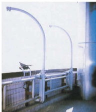
TRAVELLING DAVIT MAST
